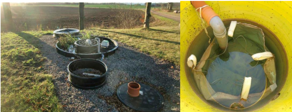
Figure 13. The ACT wastewater treatment system. The photo to the left shows the filter well with a bag filled with Petrit E.
