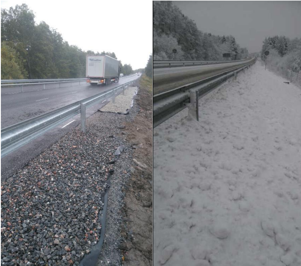
Figure 17. The RSF with crushed gravel in the foreground, followed by that with AOD-slag (left picture). Winter conditions (December) at the RSF site.
