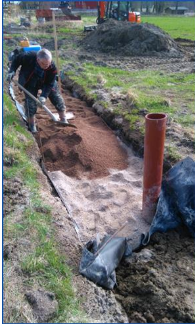
Figure 16. Construction of filter bed. The grey material in the trench is "masgrus", AOD-slag. This phosphorus-binding layer is covered by sand (red-brown color) on which the distribution pipe from the septic tank will be placed. The red-colored pipe that stands out connect to a perforated pipe in the bottom of the filter bed, which transports the treated water out to the receiver (ground water or open ditch).
