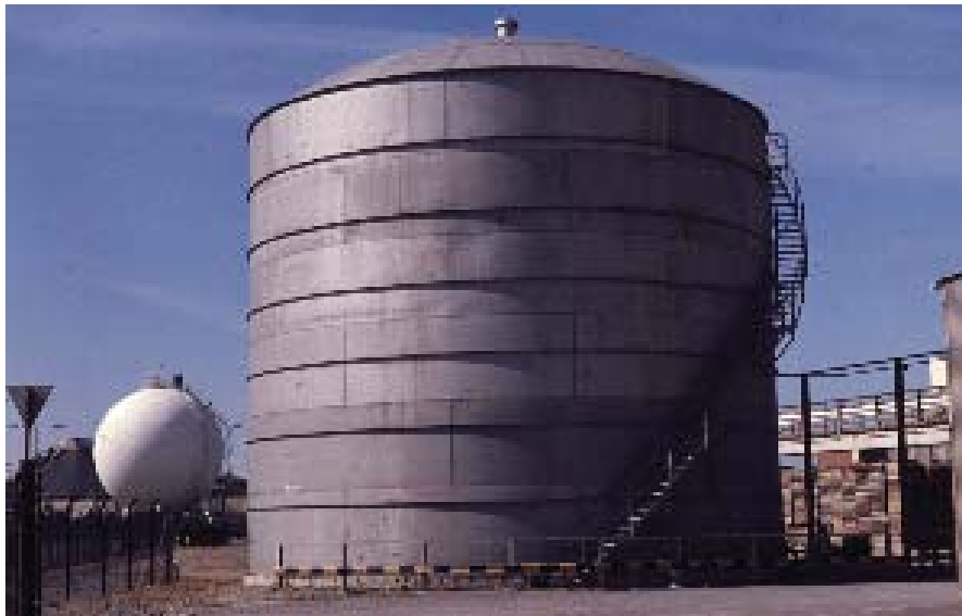
Figure 4.10 Storage tank in stainless steel.
